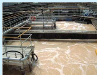
The Kuraray Saijo Plant's wastewater treatment facility utilizes the system
